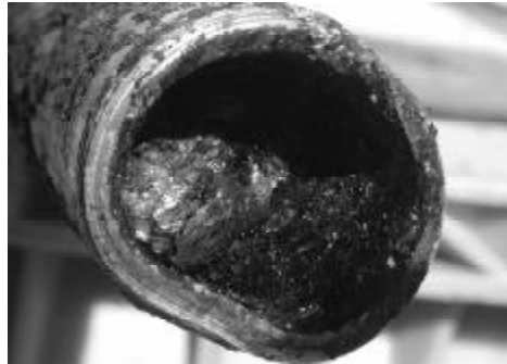
Figure 9. Closeup of vent pipe pluggage.
