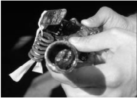
Figure 8. Plugged 1-inch vent pipe.
