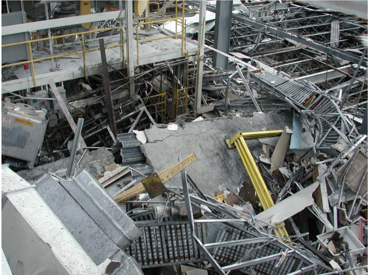
Figure B-2. Area between mixers #1 and 2. (Note upward heave of broken concrete floor.)
