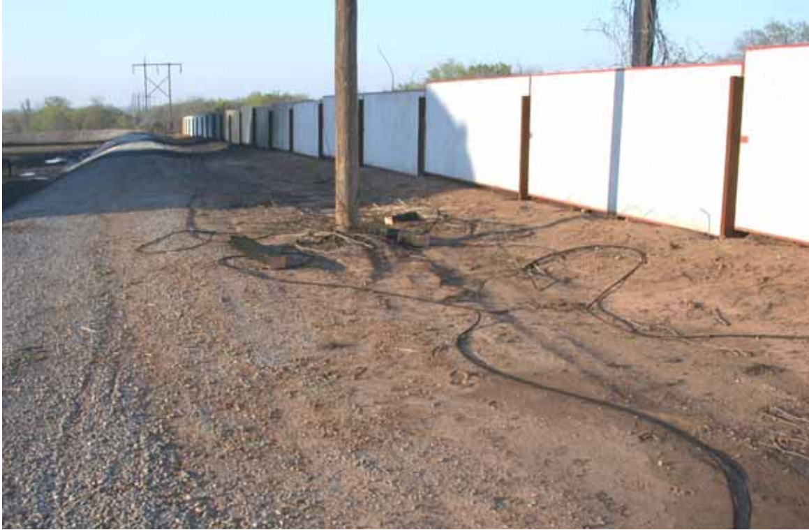
Figure 4. View of downed AEP power lines on east dike wall.
