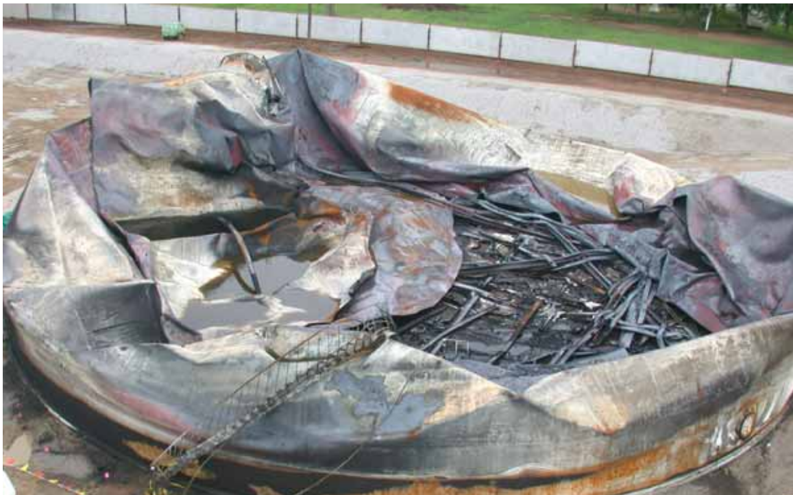
Figure 3. Wreckage of tank 11.
