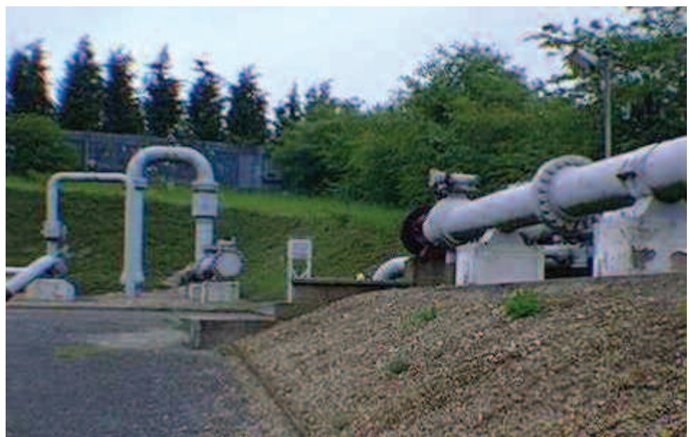
Figure 3 Surface pipelines within an oil fuel depot
