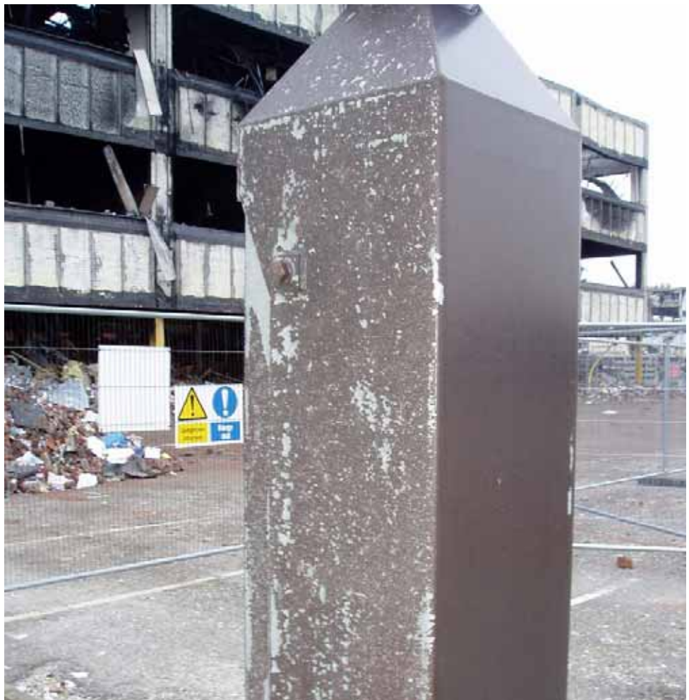
Figure 15 Steel post in the west car park of the Northgate building. The post shows abrasion marks on its south face
