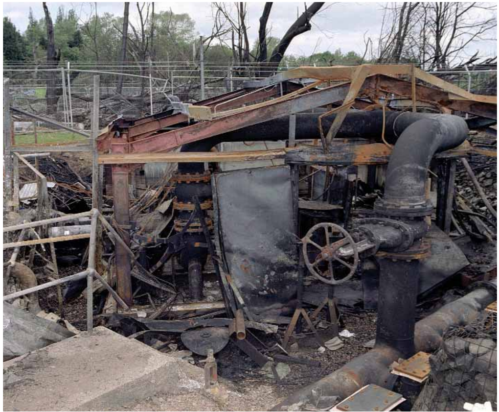
Figure 14 HOSL West emergency pump house from the south-west side. The line of trees behind marks Cherry Tree Lane
