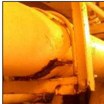
A typical pipe support detail showing “hidden” corrosion
