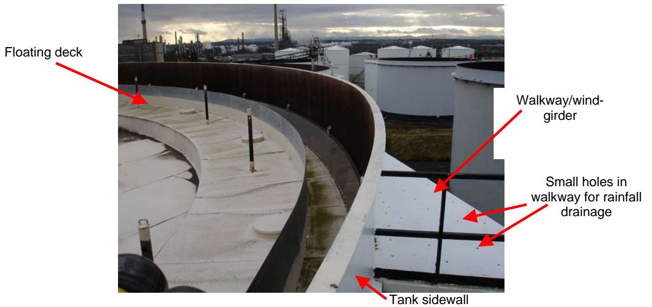
Figure 9 View from the walkway around the top of an FD tank showing the floating deck towards the top of its travel.
