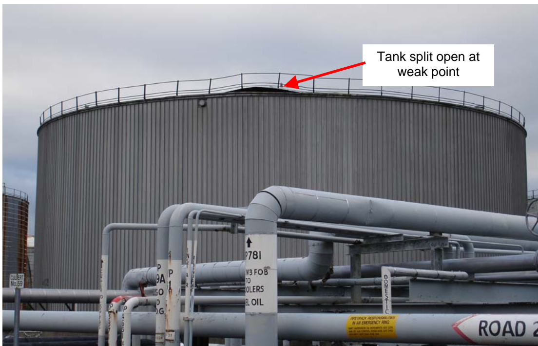
Figure 7 Photo of a fixed-roof tank that has failed around the upper rim.
