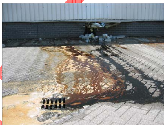
Image 11B: Integrity of compartment is compromised by falling racks
